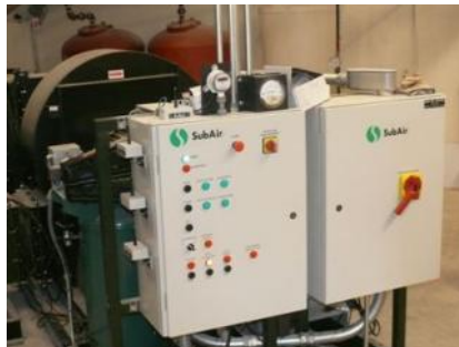
SubAir System controlling air and moisture of turfgrass on BMO Field.
